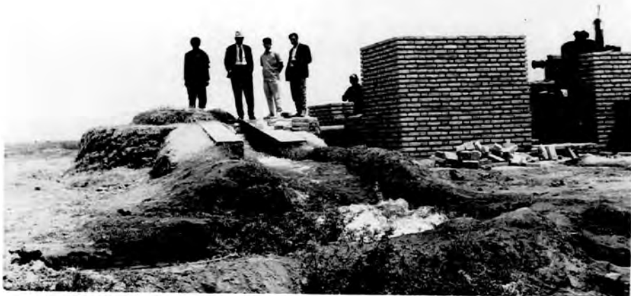
The final stage of a new electrically powered pump and its building on the Khiaban complex.
