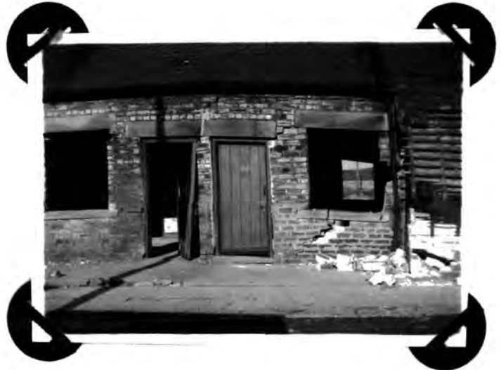
Damage caused by subsidence.
