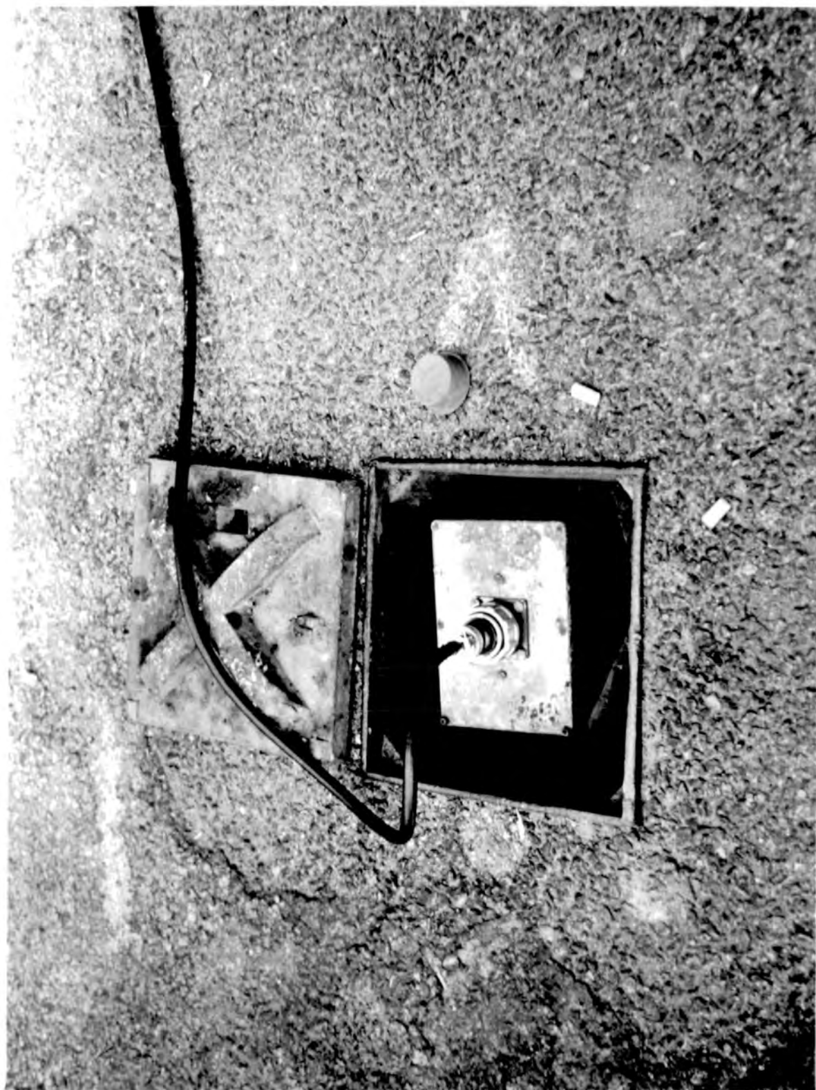
PLATE 4.1 BOREHOLE TERMINAL BOX
