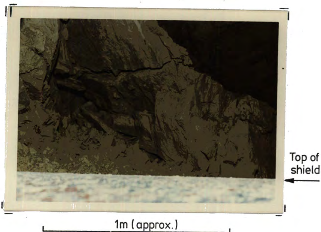
Plate 5.2 LOOSENING AND OVERBREAK ABOVE THE TUNNELLING SHIELD.
