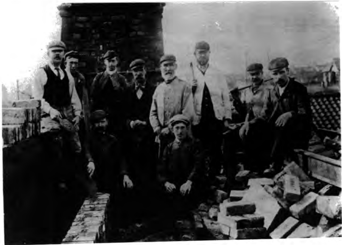
PLATE 22: a. Top PLAN AND SECTION OF BEEHIVE OVENS b. Bottom WORKMEN REPAIRING WATERHOUSES OVENS (c.1912)
