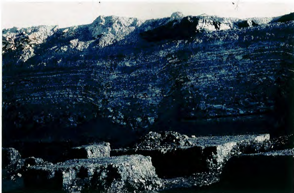
Plate 2 Coal pillars due to previous pillar & stall mining lie exposed at bottom of cut. Subsidence features related to old mine workings are exposed in cut wall.
