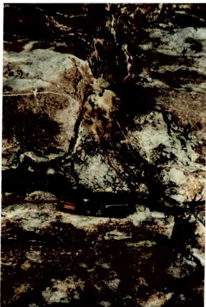
Fig. 4.59 Section through a fissure in east Sully Bay. The fissure connects with a horizontal cavity 0.5 metres below the limestone surface and contains brecciated limestone at the base of the fissure.
