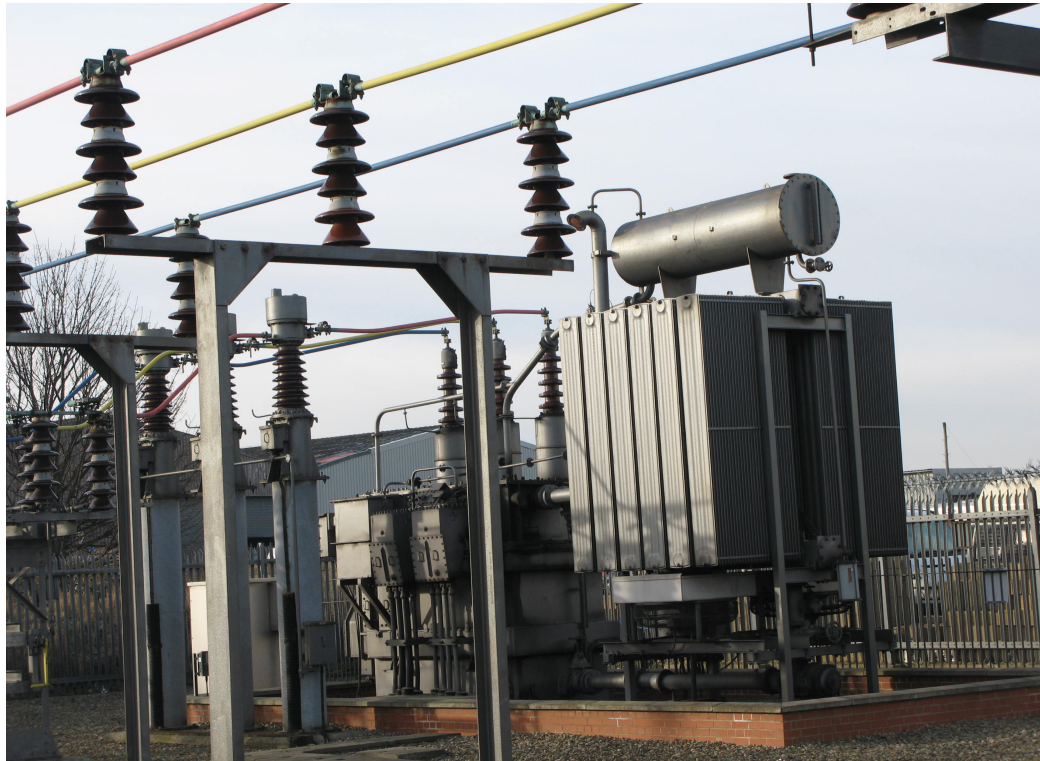
Figure 9.3 – Transformer and 66 kV busbar at Brenda Trading
