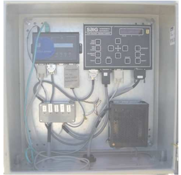
Figure 3.14: Inside the electronic cabinet. Starting from the upper right side and proceeding clockwise one can clearly identify: server, CCD controller, power supply unit and connection box. Extracted from Le Gallou (2005).
