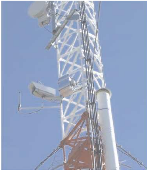
Figure 3.9: The transmitter mounted at Gamsberg's telecommunication mast. One can see the antenna, light emitter and the water tank (left to right). From Le Gallou (2005).
