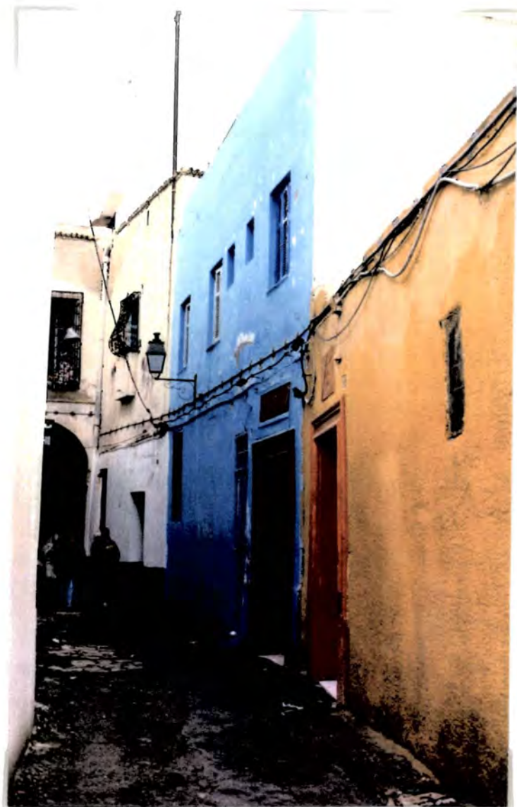
Plate 35: Aesthetic issues: multi coloured renderings take the place of traditional whitewash on the facades the buildings of the Medina, in this case on the Rue Sidi Ali Ben Diaf, January 1991.
