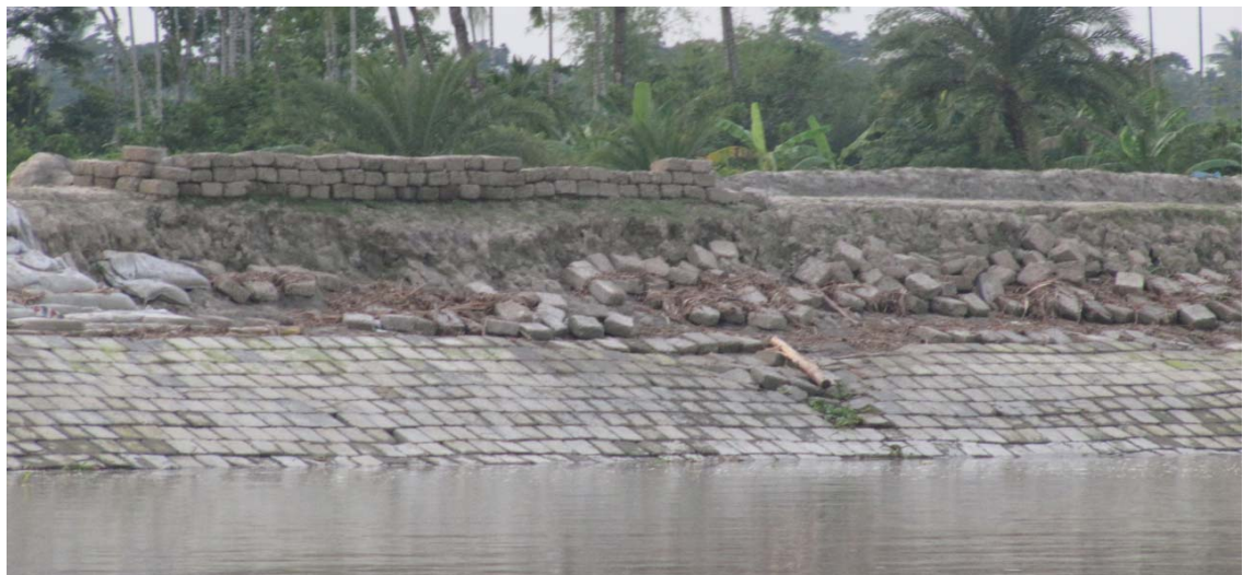
Figure 4.2: A damaged and poorly maintained part of embankment in the Sarankhola Upazila
