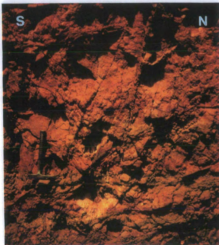
Photo 4.4.7- Continuous to quasi-continuous fractures centimetre-scale to metre-scale spacing typical of the Bahia Mine exposures.
