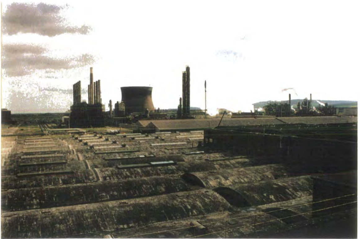
Figure 3.1: The roof of the Melinar Stores, ICI Wilton, Teesside. Upper photograph looks south-west and shows the main level of the roof with the derelict polypropylene production unit in the background. Lower photograph looks north-east, was taken from the polypropylene unit and shows the main level of the roof.
