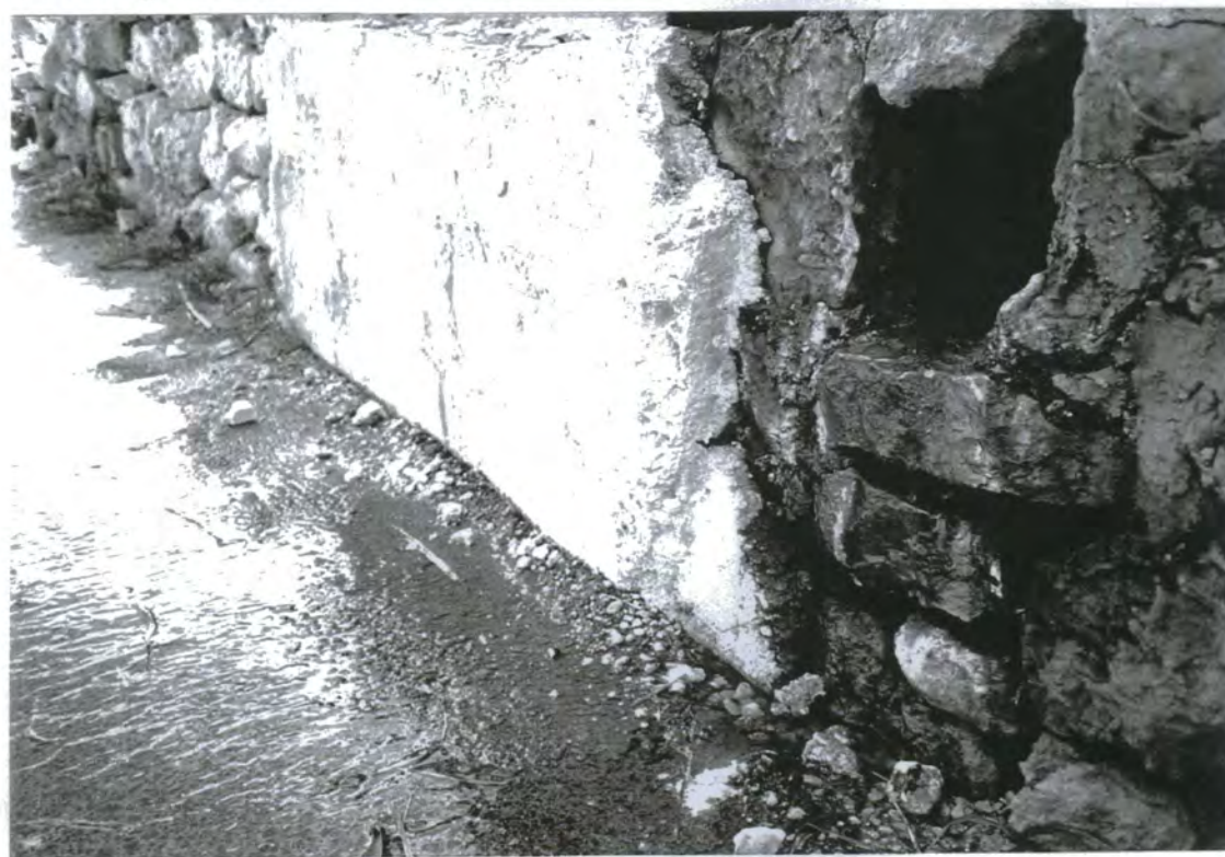
Plate 5.6. Large volumes of water leaking from a water channel. It can take several days before it is reported and repaired.
