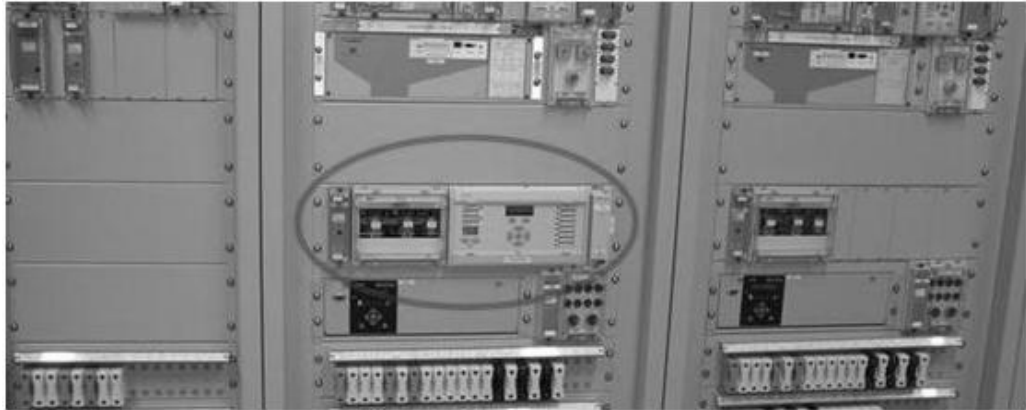
Figure 54: Substation relay user interface
