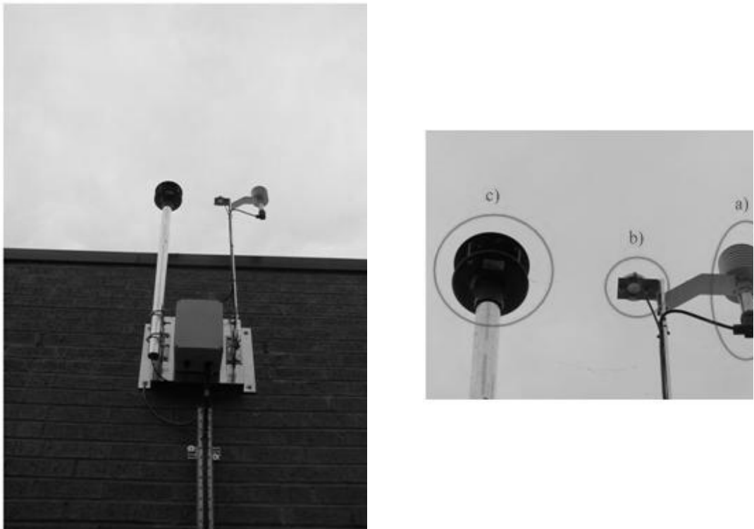
Figure 53: Meteorological station in a distribution substation and particular. a) pressure sensor, b) solar radiation sensor, c) wind speed and direction sensor
