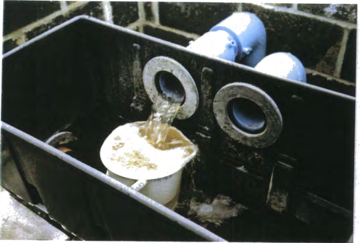
Plate 3. Wastewater inlet tank at the CATS Terminal reedbed, January 1997, showing secondary treated effluent entering the system from the Klargester.
