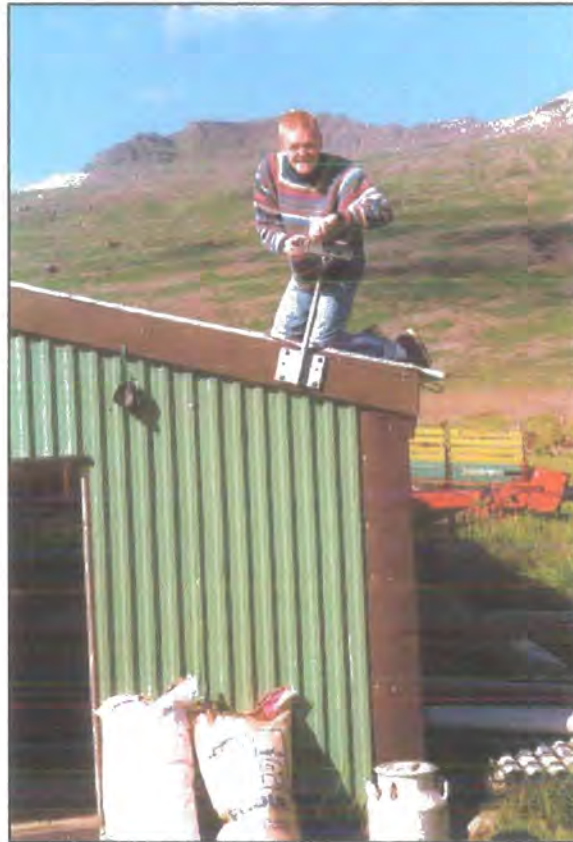
Figure 3.7 Installing the GPS antenna on the roof of a building at station HOT19 (Fell).
