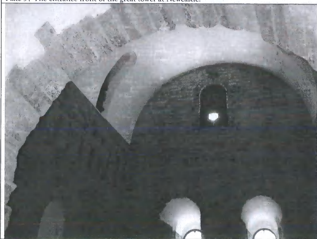
Plate 58 The roofline at Newcastle showing the gallery at third floor level above it.
