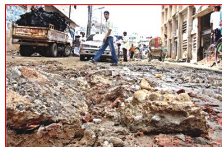
Figure 7.5: Road digging: A symbol of non-coordination
