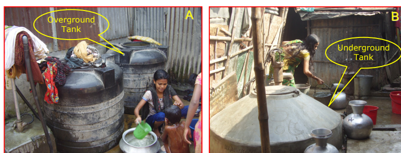
Figure 6.12-A,B: Communal water storage facility
