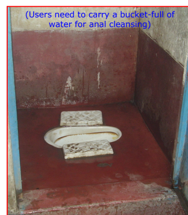
Figure 5.3: Absence of water source inside the latrine
