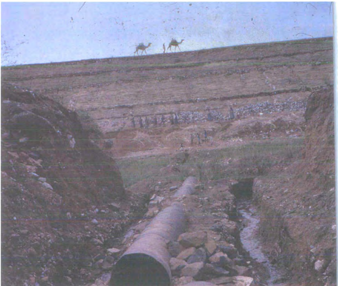
Plate 4.1. The seepage area and the dam embankment seen from below.
