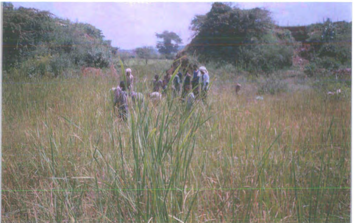
Plate 5.1. Seepage area below the dam being drained (above) and shortly afterwards- reeds maintained and access prohibited to cattle and people (below).
