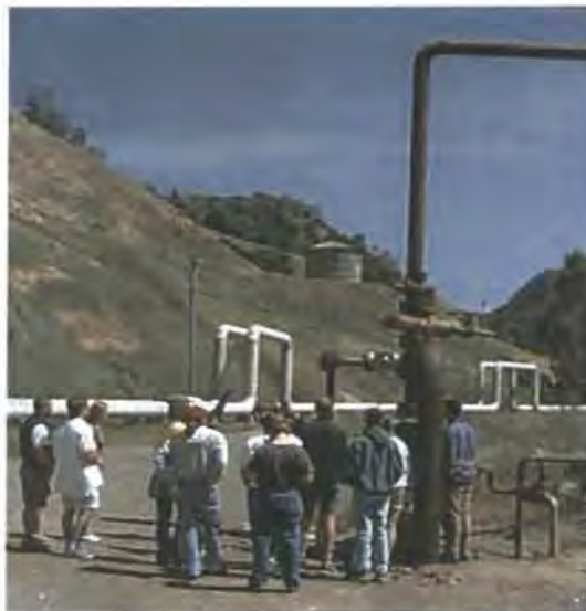
Figure 1.28: An injection well at The Geysers geothermal area. Most injection wells are located in the vicinity of the power plants. (from : http://corporate.stanford.edu/research/programs/geoth.html )
