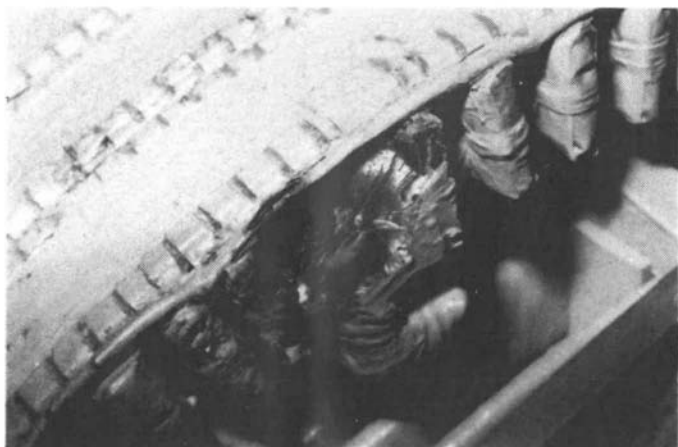
Fig. 10 Damage to the wound rotor of a 4.8 MW induction motor detected by gas monitoring
