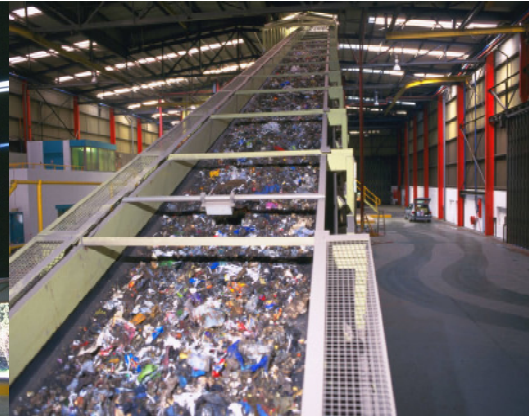
Figure 1.9: a hopper, transporting MSW from the shredder to the digester tower.
