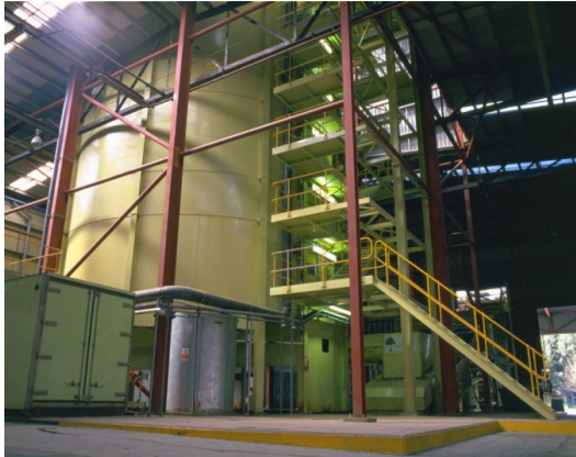
Figure 1.8: a PWM digester tower
