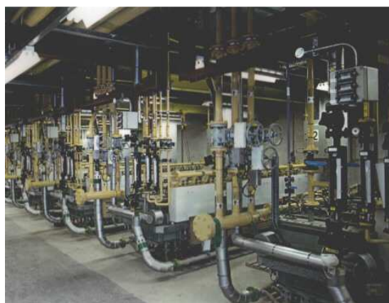
Figure 3: Fluorine cell room at F2 Chemicals Ltd., Preston
