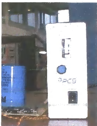
Figure 4.57 -Signal Conditioner - The pump outlet pressure transducer control
