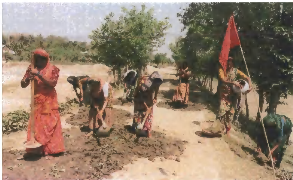
Figure 5.2: The RMA women are maintaining the rural earthen roads to keep it passable year-round (Photo: RMP/CARE)
