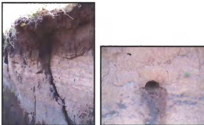
Figure 4.15: Evidence of bank erosion from desiccation cracks and burrowing animals.
