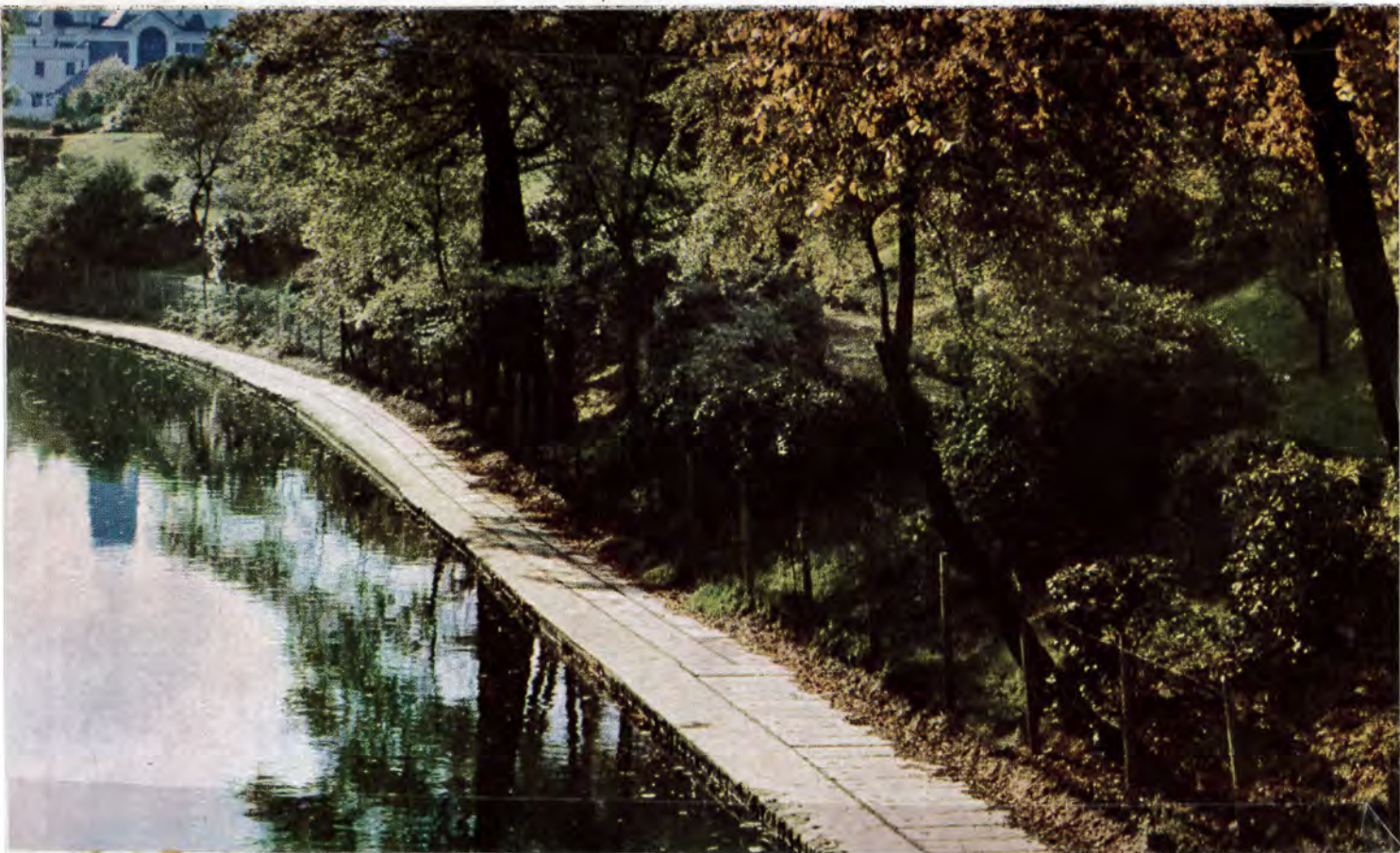
Photograph 27. Towpath of the Grand Union Canal through Regents Park, London, showing concrete covers to the 275 kV cable troughs.
