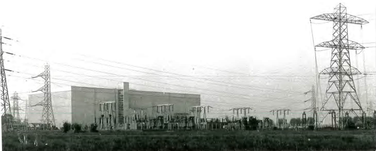
Photograph 39. Whitson 275 kV switchhouse was the first switchhouse of this size, and is typical in size and appearance to many others built in exposed situations or on restricted sites.
