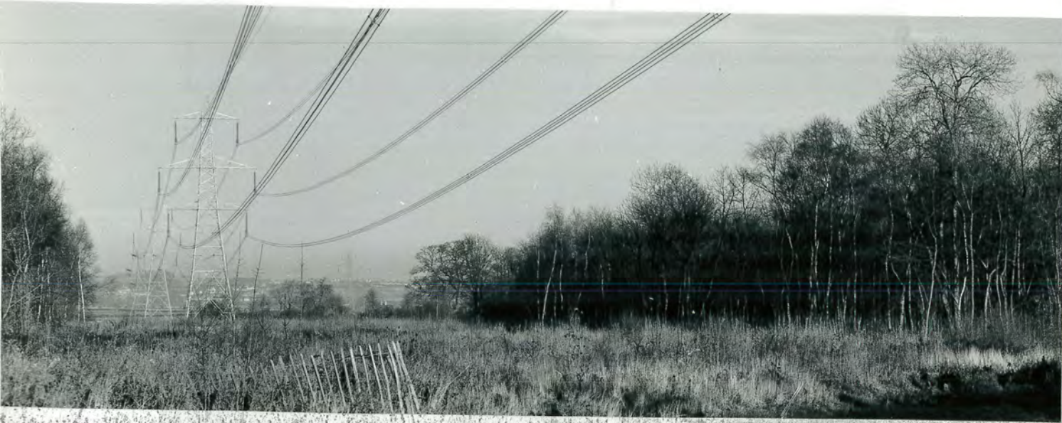
Photograph 20. The last span of a 400 kV line into Cowley substation near Oxford. This clear felling has opened up a view into the substation, behind the photographer, from a road in the middle distance. This could possibly have been avoided if a few trees had been retained near the tower. The trees at the edge of the swathe, being formerly in the heart of the wood, and thus tall and slender, are very liable to be blown over in a high wind. See next photograph for view in opposite direction.
