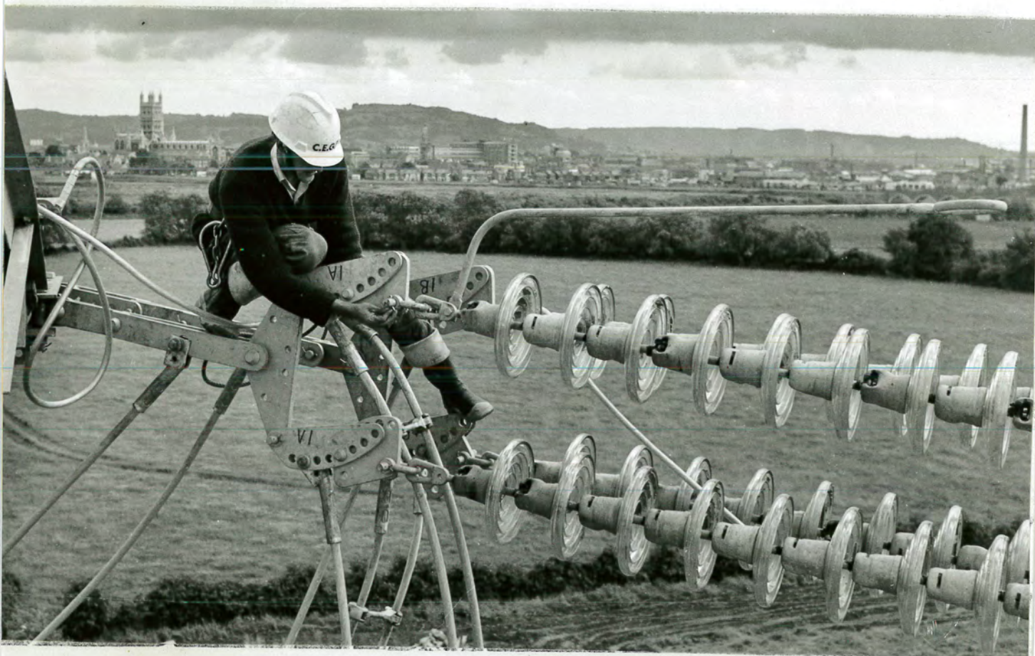
Photograph 66. A tension string of four, 400kV glass insulators, at the Gloucester end of the line to Ystradgynlais substation in South Wales.
