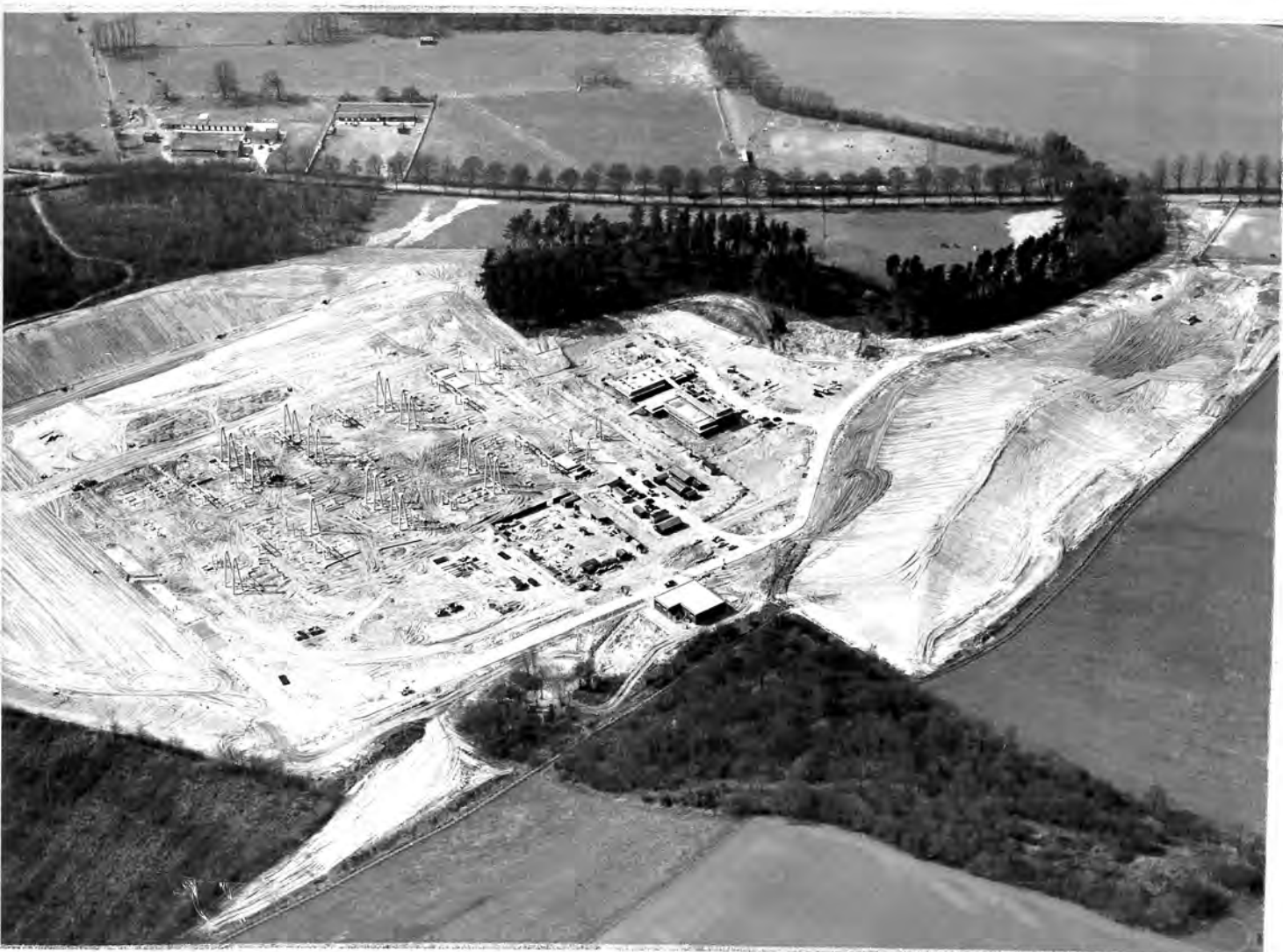
Photograph 76. Air oblique view of Hurst 275/132 kV substation looking westwards. London Borough of Bexley. M.R.489730. This photograph taken on Wednesday, 9th April 1969 shows the substantial completion of the preliminary earthworks just prior to grass seeding. This site is generally regarded as being a very good one from a visual amenity point of view as the substation has been carefully located between Sands Spinney to the top right of the photograph, Cavey's Spring in the bottom right, and a Forestry Commission Plantation on the left. The only vulnerable aspect was to the east of the site where land modelling 40 ft. high has been carefully designed and shaped to provide a line of visual cut off for the occupants of dwellings further to the east. Planning permission required a landscaping scheme of which the ground modelling formed the first stage. The second stage tree planting will be carried out next year in order to clothe the new land form, and to complete the screening of the whole site. The care taken in site selection and landscaping will help to ensure that when the substation is finished it is unlikely that any of the local residents will even be aware of the existence of this major switching and transforming station in their neighbourhood.
