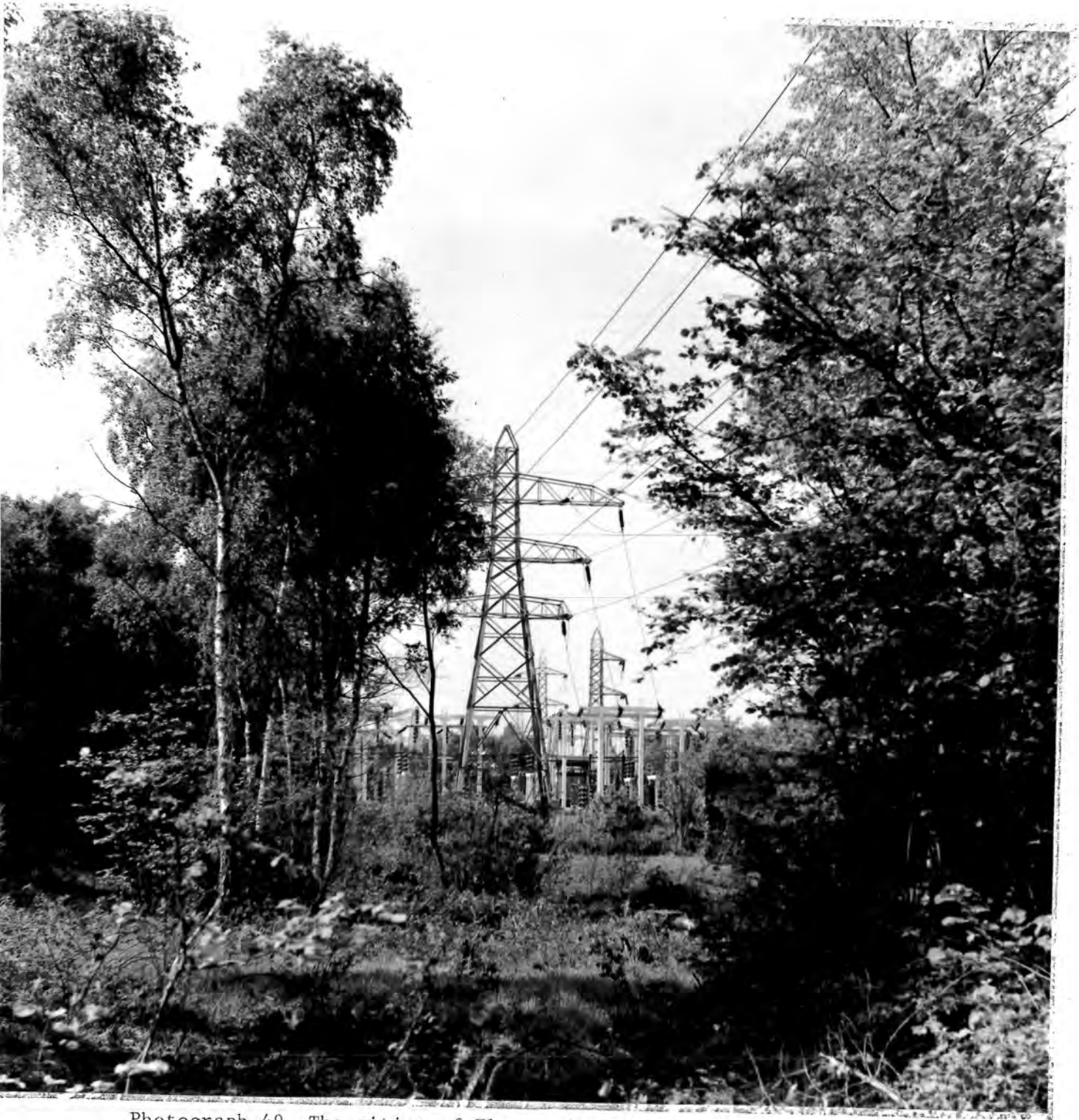
Photograph 49. The siting of Fleet substation in Coxmoor Wood has provided complete and effective screening from all public viewpoints. This view was taken within the wood in a small area cleared to permit erection of the overhead line.
