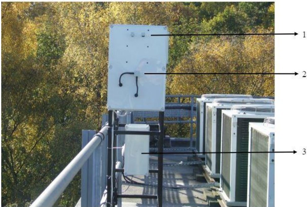
Figure 3.11 Installed view of transmitter
