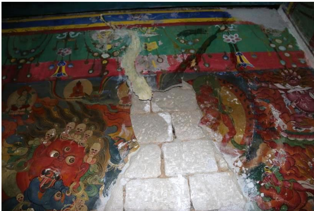
Figure 2.8: Mural paintings within the Dubdi Monastery in Yuksom, West Sikkim, damaged by the 2011 Sikkim Earthquake (Image Kai Weise).
