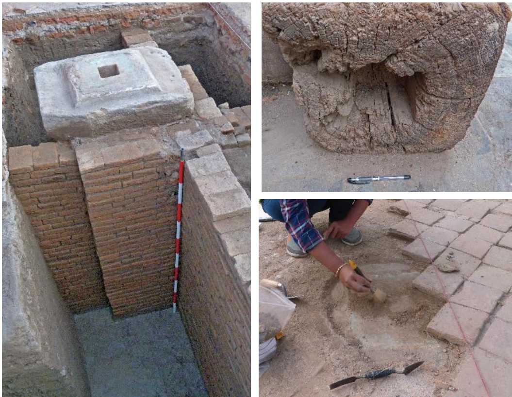
Figure 6.10: The brick in mud mortar foundations piers in perfect condition and the deteriorate base of a central post missing a tenon, and the saddlestone covered with flooring tiles (Images UNESCO Chair, Durham University).
