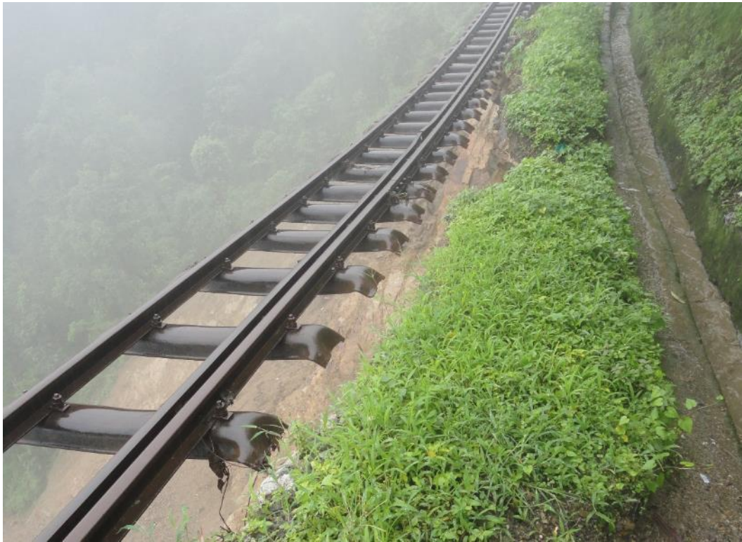
Figure 2.7: Suspended tracks of the Darjeeling Himalayan Railway, a World Heritage property, due to landslides caused by earthquake and heavy rains (Image Kai Weise).
