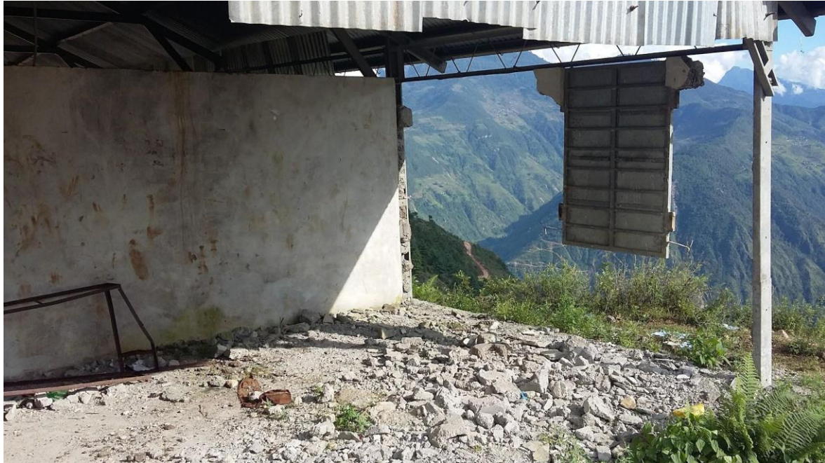
Figure 5.4. In Listi, a building lost most walls in the earthquake while a window-shutter holds on (Photo credit: author, 2017).
