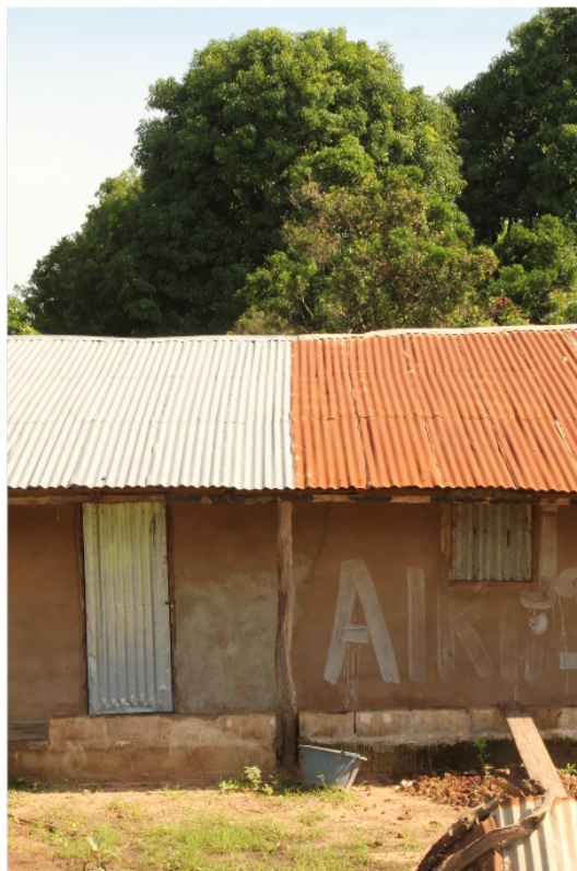
Figure 4. 1 A new (left) and rusted metal roof (right) in a Gambian village. (Lindsay, S., personal collection).
