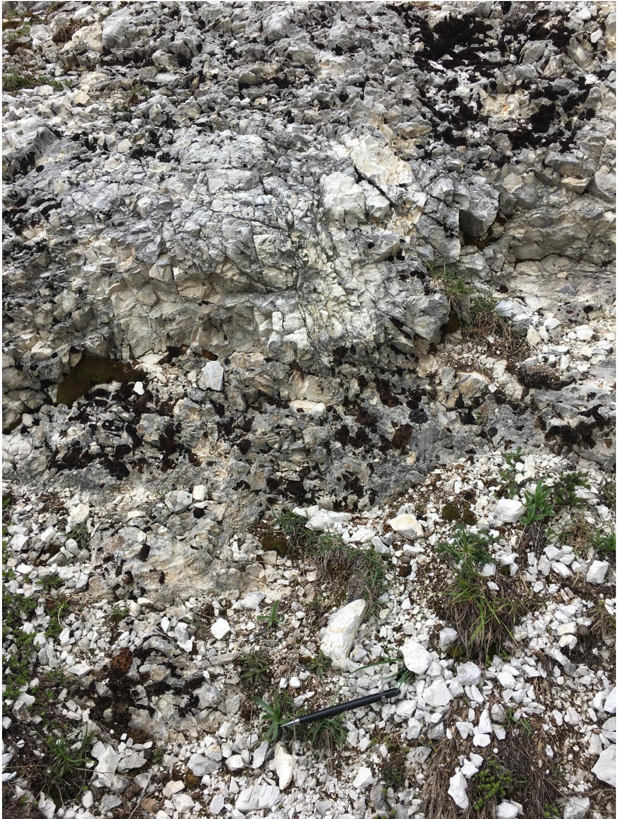
Detail of scarp deterioration and hanging wall debris (pencil for scale)
