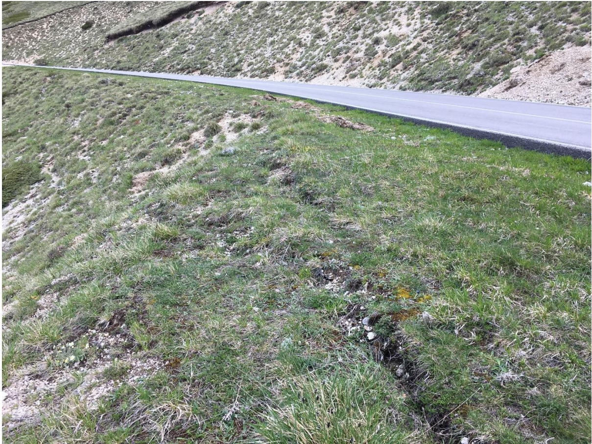
Cracks in slope on hanging wall side, looking W
