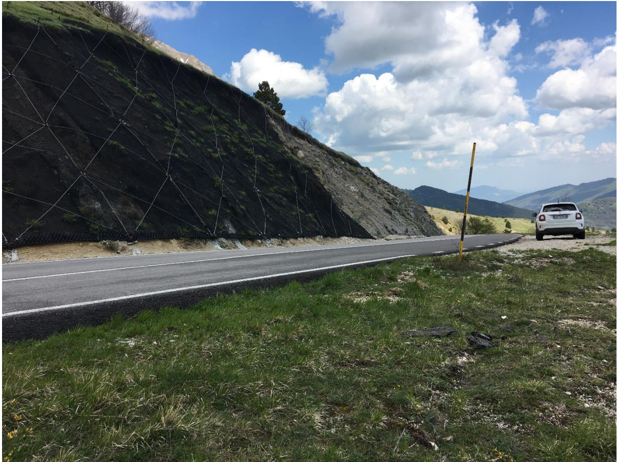
Cracks in slope on footwall side, looking ENE
