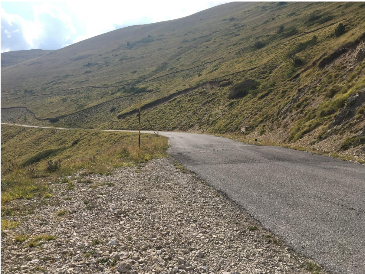
Figure 121: Vettore Road site photograph taken on 27th August 2019, looking WSW, repaired road section to right of snow pole.
