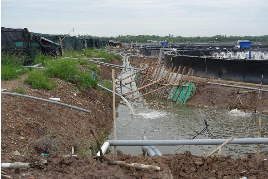
Figure 35 Shrimp ponds, pipelines, and wastewater
