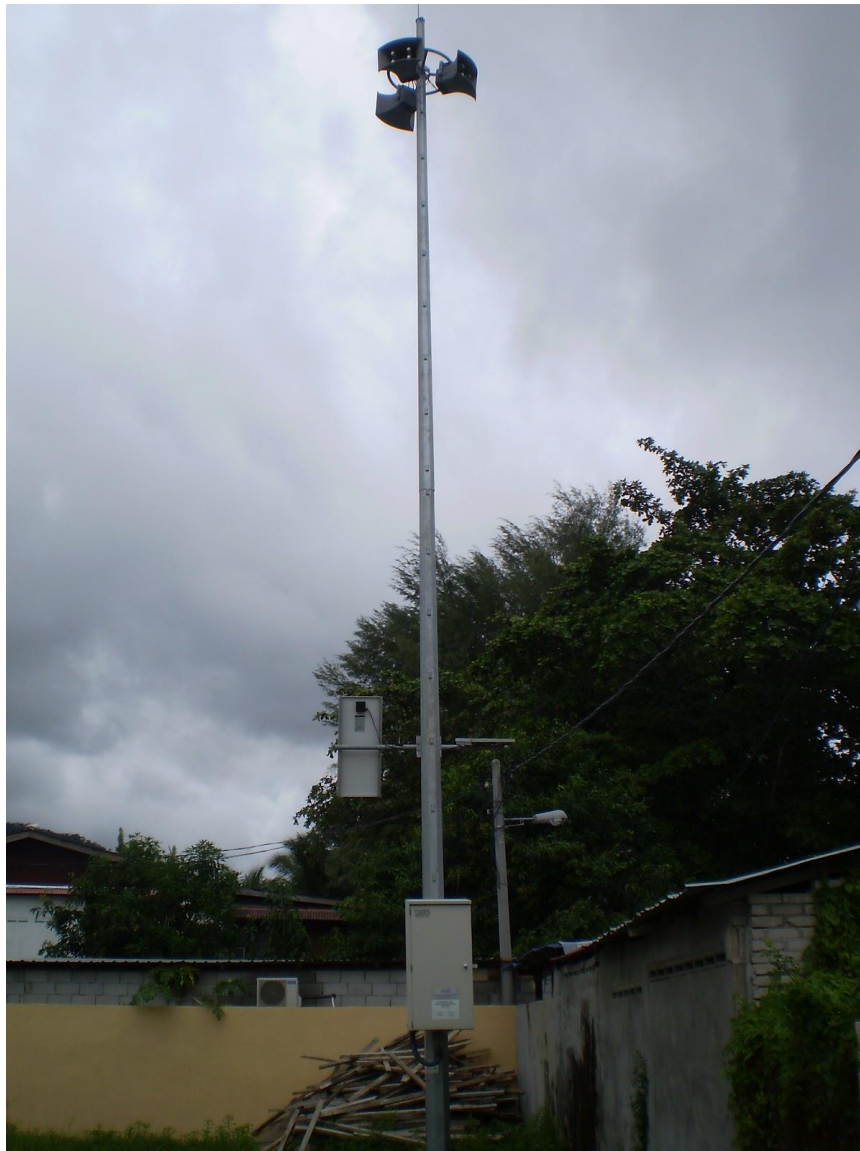
Figure 6.8: The only emergency warning siren installed in Teluk Kumbar.
