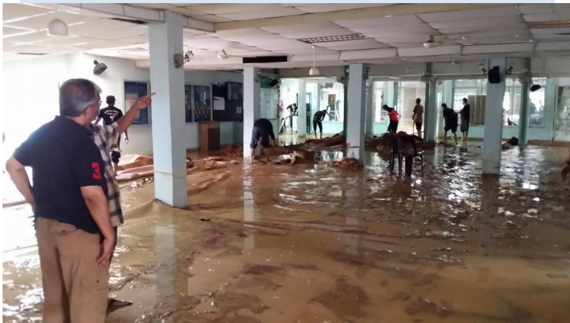
Figure 6.8: Teluk Kumbar Community Hall: Impact of flooding
