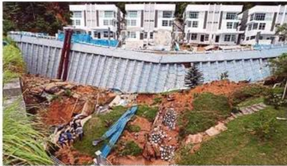
Houses damaged by the landslide in Tanjung Bungah, Penang. PIC BY MUHAMMAD MIKAIL ONG
