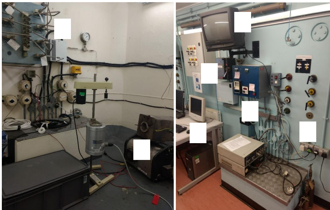
Figure 9.5. Inside an example cell (left) and the control room (right) of Durham HPL
