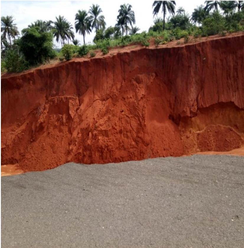
Figure 7.1: Destroyed connecting road linking Asaa & Obibi-Ochasi communities.
