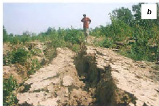
Figs. 2.07a-b: Extensional cracking and liquefaction-induced cracking from the Kutch Earthquake in India in 2001. Full credit to Rajendran et al. 2001 – reference in bibliography. Digital enhancement of the images has been tried, but to no avail as this is the quality at which they were initially published.
