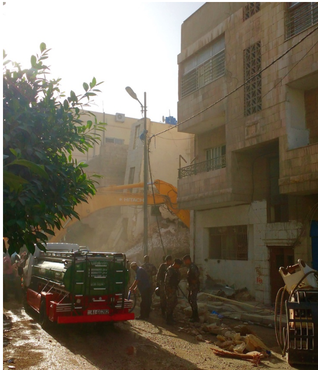
Fig.12 Building Collapse, al-Ghawariyah
