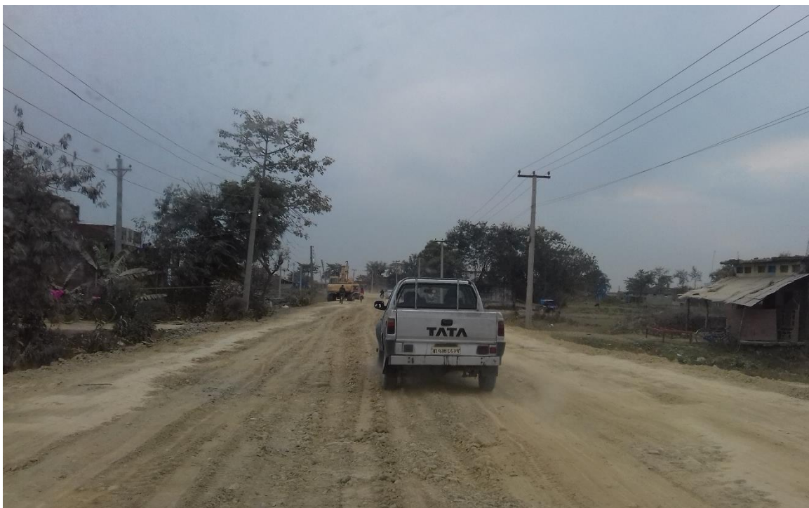
Figure 6.2 : On-going roadwork, funded by ADB through SASEC, on the Lumbini-Taulihawa stretch to extend the road from two to four-lanes
