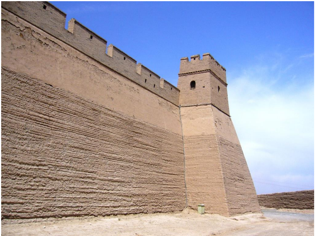
Figure 2.1. Rammed earth portion of The Great Wall of China at Gansu, China. Photo retrieved from https://www.murailledechine.com/voyage-jiayuguan-gansu
