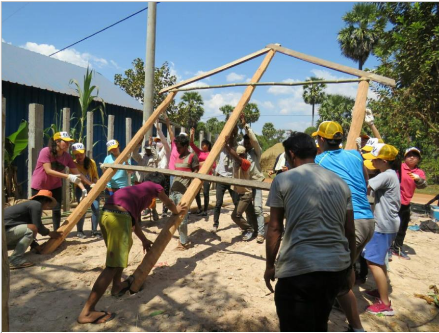
Figure 11 Everyone having their hands on the structure of the house at the moment of lifting it up
