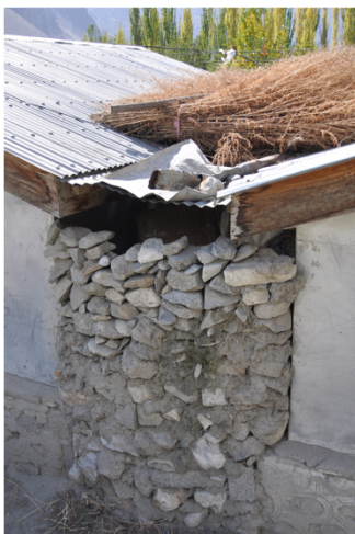
Coarse stone masonry wall constructed between shelters to protect items in Aliabad.
