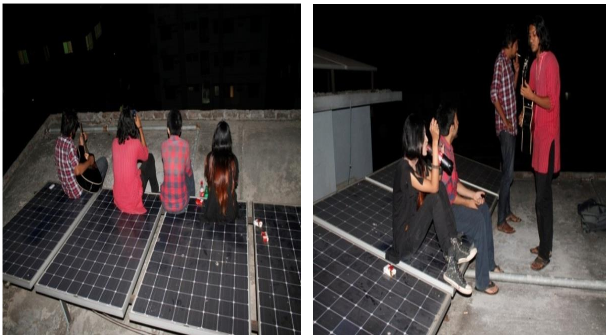
Figure 8:9 Out of service solar panels Source: Author
