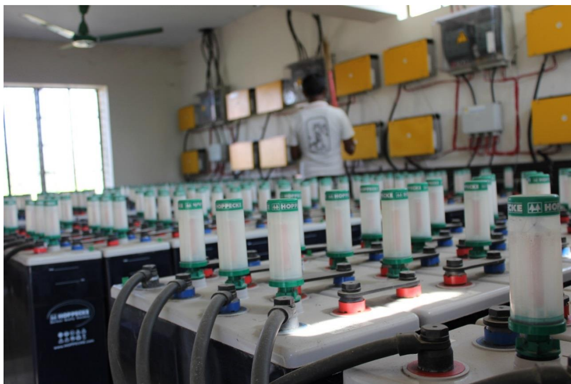
Figure 6:11 Inside Purobi mini grid power station
