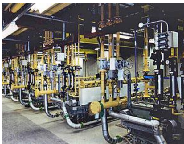
Figure 7 Fluorine cell room used in the manufacture of perfluorocarbon gases and fluids, at F2 Chemicals Ltd, Preston, UK
