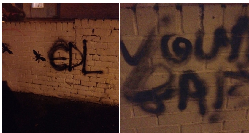
Figure 5.3: Graffiti on the walls of the HIDE2 yard
