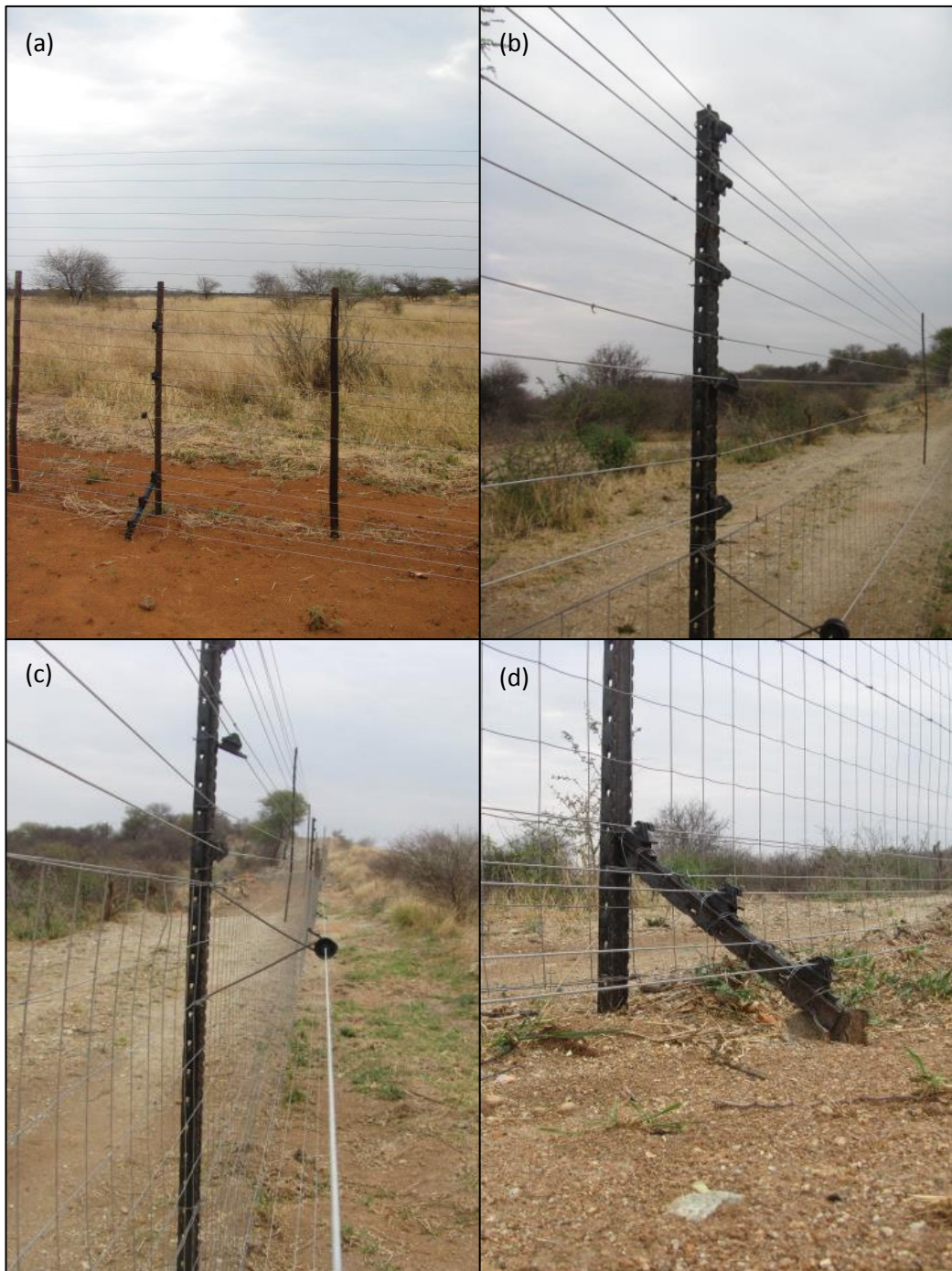
Figure 13: (a) Fence is 2.4m high. (b) Five electrified wires at the top (identified by the black plastic insulators on the droppers), each separated by a non-electrified wire. (c) One electrical wire offset at a 45° angle to the fence. (d) Three electrified wires at a 45° angle to the fence, each separated by a non-electrified wire.
