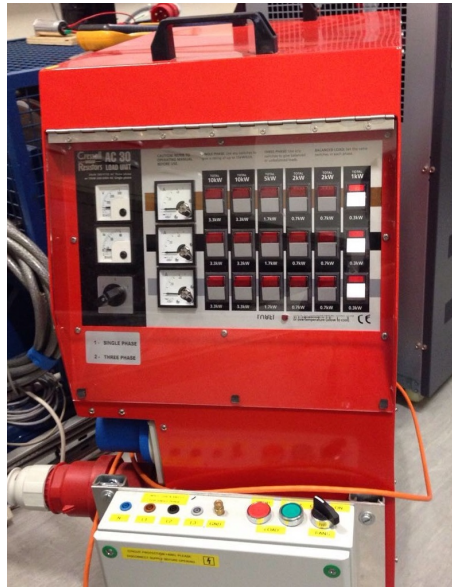
Figure 6.2: The high power load bank used for initial controller testing with the converter.
