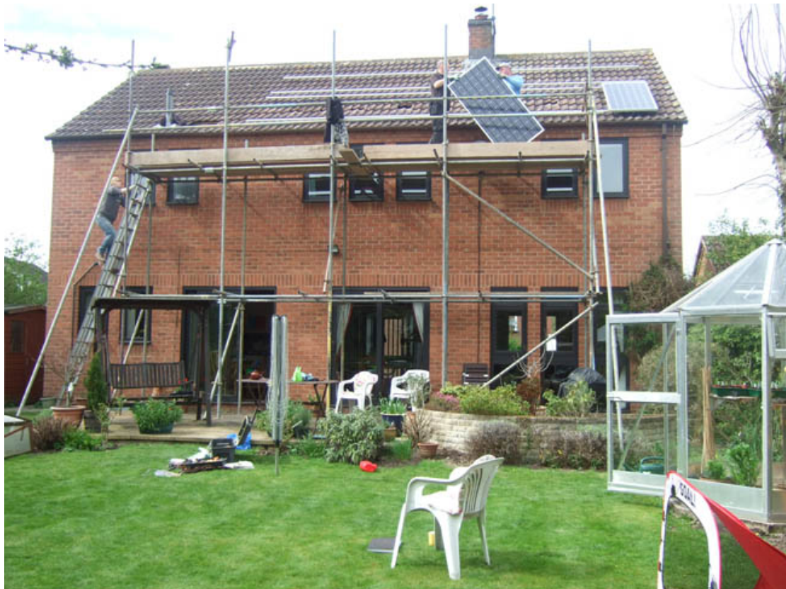
Figure 4-1: Solar installation at Peter and Anne's home, April 2011
