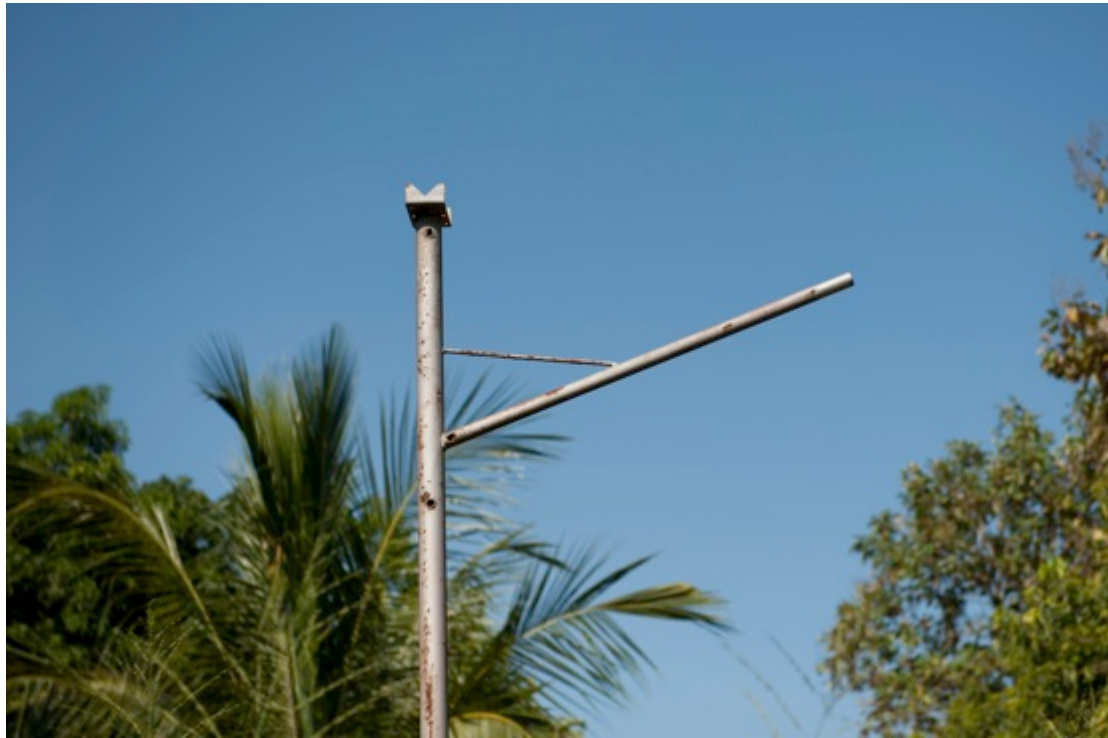
Figure 6-2: Solar Street lamp with lamp, panel and battery removed, Galgamuwa, Sri Lanka
